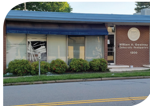
The Democratic Headquarters in downtown Little Rock was damaged during protests on the night of May 31.
